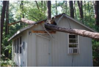
Photo above: Cabin #10 at Camp Occohannock damaged during Hurricane Irene. Volunteers needed to help clean up uprooted trees and repair the cabin. Contact Camp Director Jerry Mobley at 757-442-7836 or email him today at <ootbay@verizon.net> !
